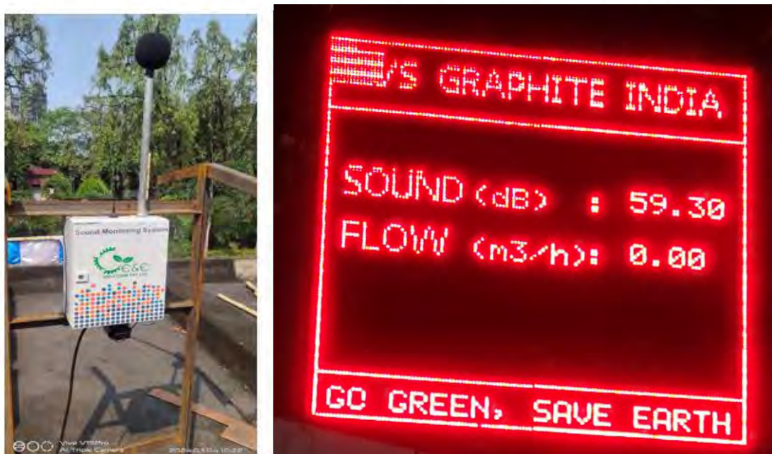
For EC compliance Ambient Noise level Monitoring Station Installed – Commissioning is in process
